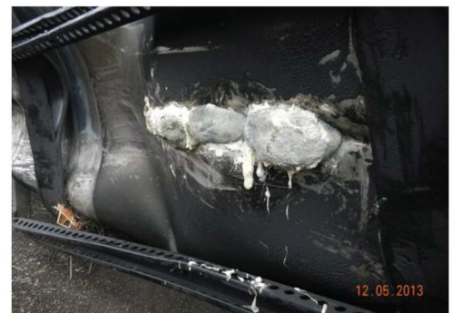
Another actual incident on Dec. 5, 2013. Three Footballs and four Golfballs needed to stop this leak!
